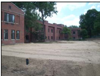
(Above) The work begins! This photo, taken in mid-July, shows the excavated Phase I construction site on the south side of The Friendly Home.
