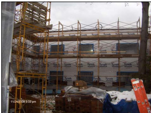
Scaffolding is in place so work can begin on laying brick on the wall facing the interior courtyard of the new addition.
