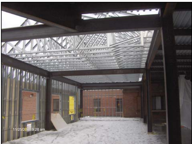
View of the roof trusses on the second floor of the new addition.
